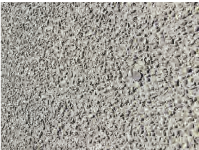
HIGH SEVERITY WEATHERING
