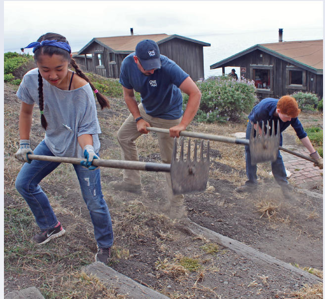
LINC summer interns help to repair the trails at the Steep Ravine Cabin site at Mt. Tamalpais State Park.
